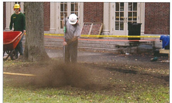
Soil invigoration leaves the soil in place and fractures it with the use of a large, supersonic air tool. Organic matter is then mixed into the soil profile.
